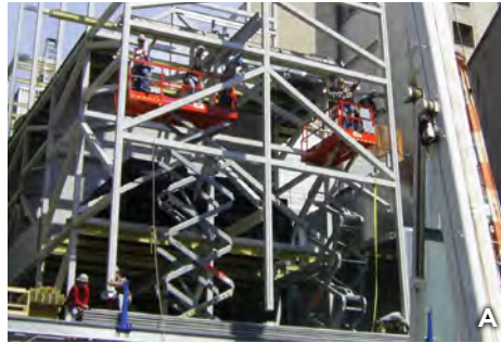
A. With CCS, safety and efficiency are always design mandates. Our exclusive structure with its large spans allows for crew members to work from the safety of scissor lifts rather than ladders.
